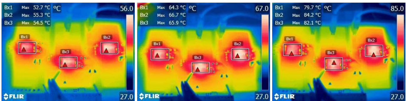
d) 100 W Inverter Output Power
